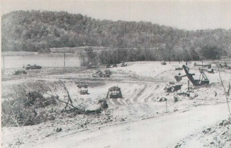
At almost every turn TVA's heavy equipment operators are busy with excavation and grading work. Some two-million cubic yards of earth must be excavated before plant is completed.
