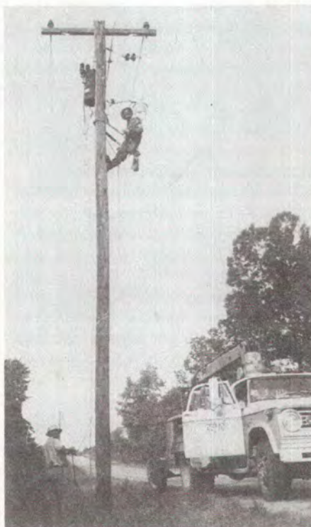
A common sight around Orlinda are Cumberland Electric Membership Corporation linemen and service trucks. The co-op has electrically served the Orlinda area for more than a third of a century.
