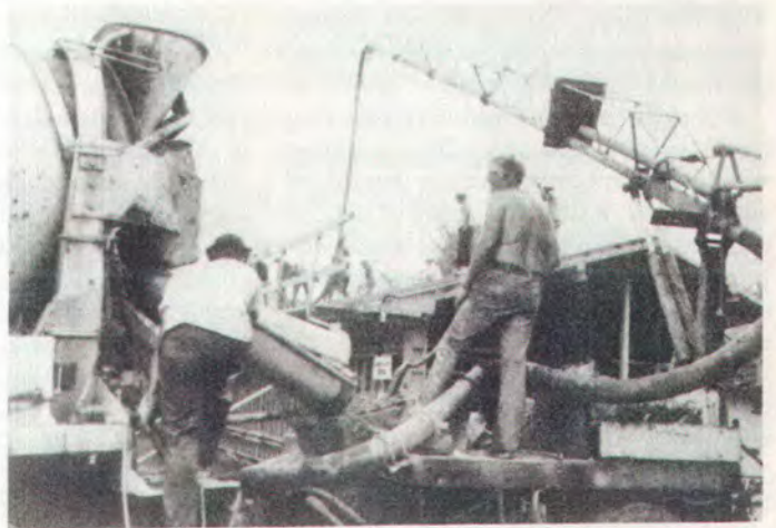
Concrete is dumped from truck into machine which pumps mixture into wall molds and onto roof.
