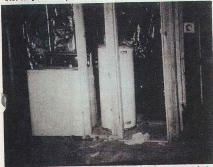
Construction begins by placing stud walls. Note good insulation behind appliances. This is a must in basement conversions.
