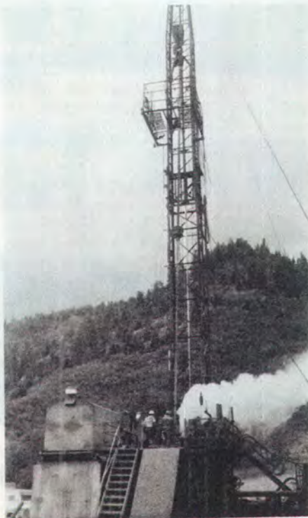
This is the drilling site of Baca VI in the Valle Grande, located in the old volcanic mountains of New Mexico about 25 miles northwest of Los Alamos. At least one area of steam has been reached in this drilling. Note height of derrick by comparing with workers standing on platform.
