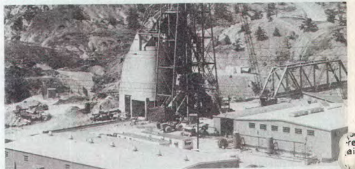
Surface facilities of the Company's newest mine are pictured here. Sinking of the shaft is complete and the shaft steel is being installed. The new mine will be known as Tennessee mine.
