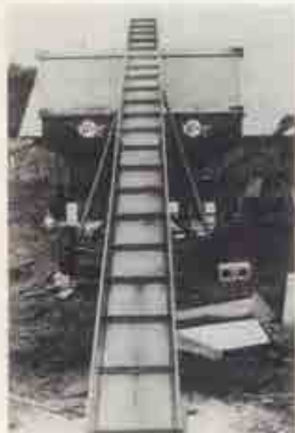
This is where the automated grain drying-storage begins. Grain is transported by way of this conveyor from the dumping pit (at bottom of picture but not shown) to 1,225-bushel holding bin at top of picture.
